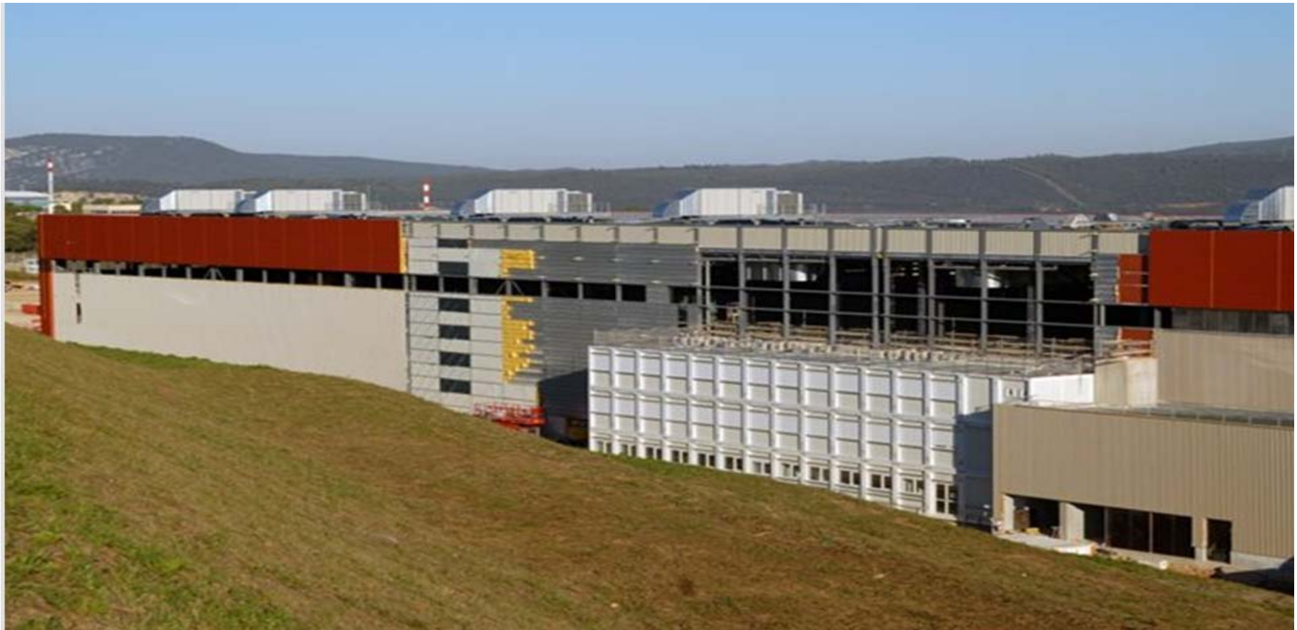
Work advances rapidly on the Poloidal Field Coils Winding Facility in August 2011: the cladding is nearly finished, the three-floor office building is in place ... Photo: F4E
