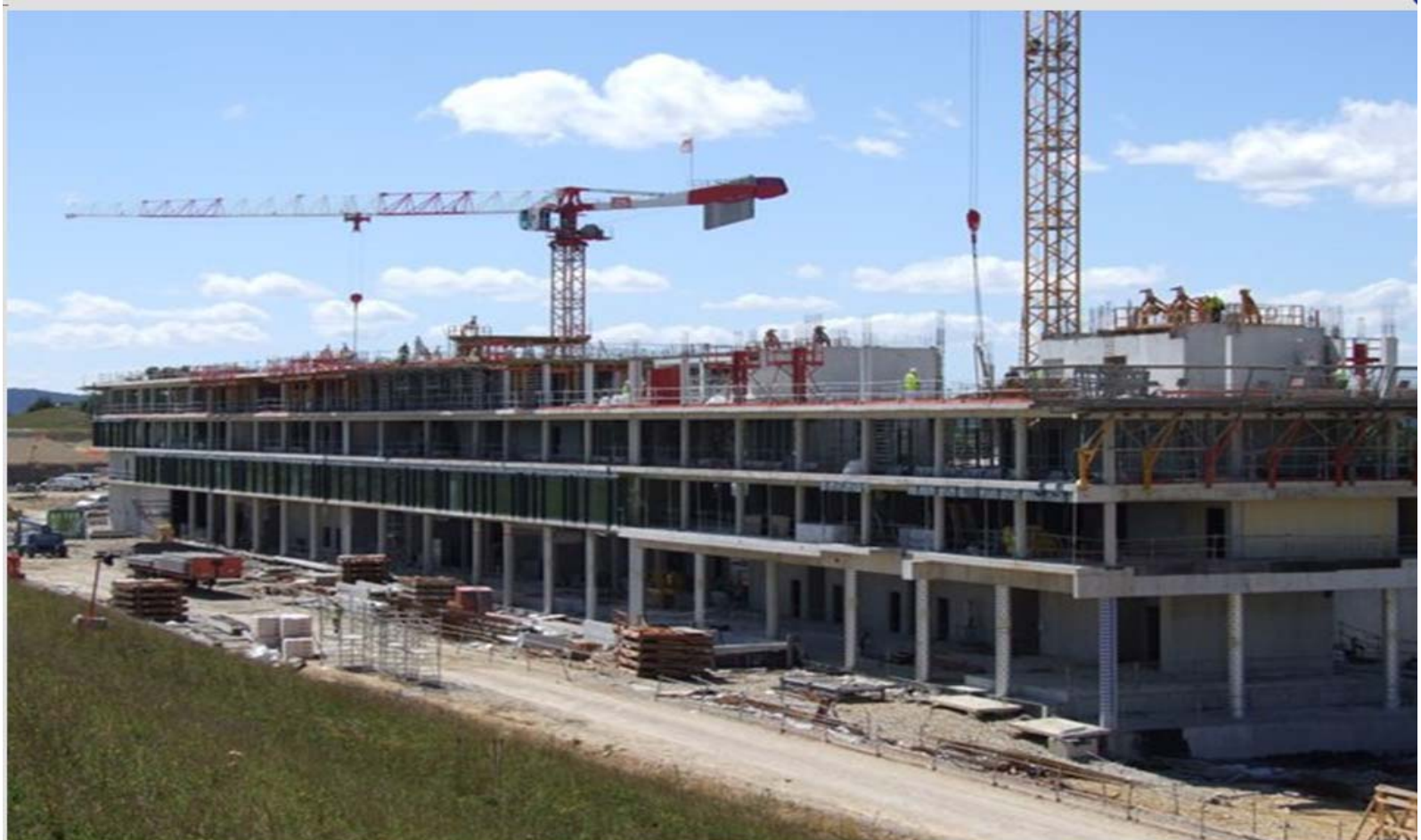
No summer break on the ITER site! Work advances on schedule on the upper floors of the future ITER Headquarters building. Photo: AIF July 2011
